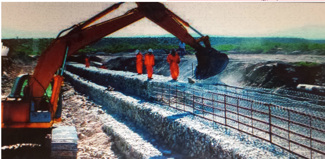
Some examples in PERU of INCA Andenes Technology used in Modern Rural Infrastructure Source: Internet; Seminario Obras por Impuestos, Lima PERU
